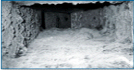
A duct before cleaning.
